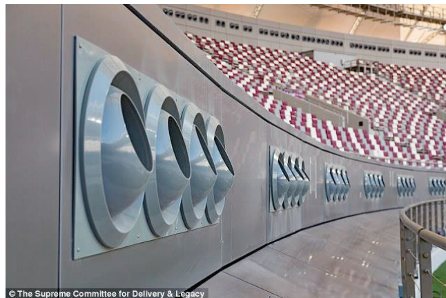
Cooling air nozzles
